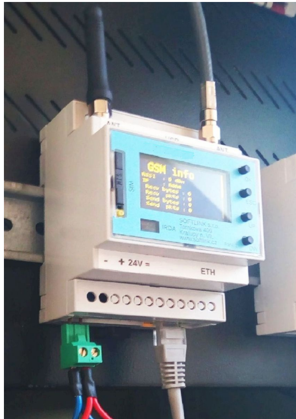
Figure 9: View of installed WL868-RFG module
